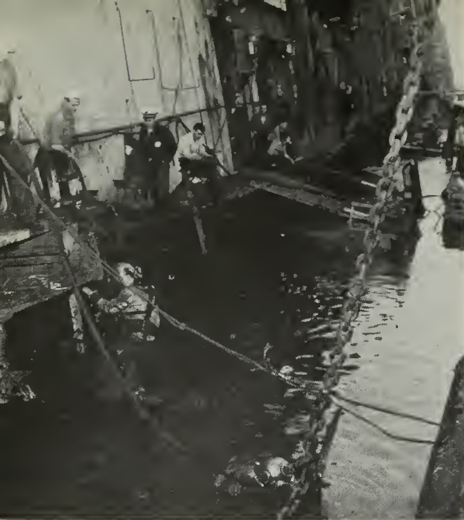
SALVAGE of USS Lafayette (ex-Normandie) in N. Y. harbor provided classroom for Navy salvage divers.
